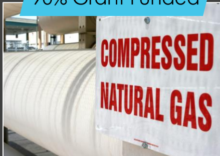
Transit CNG Fueling Equipment $6.4 Million
